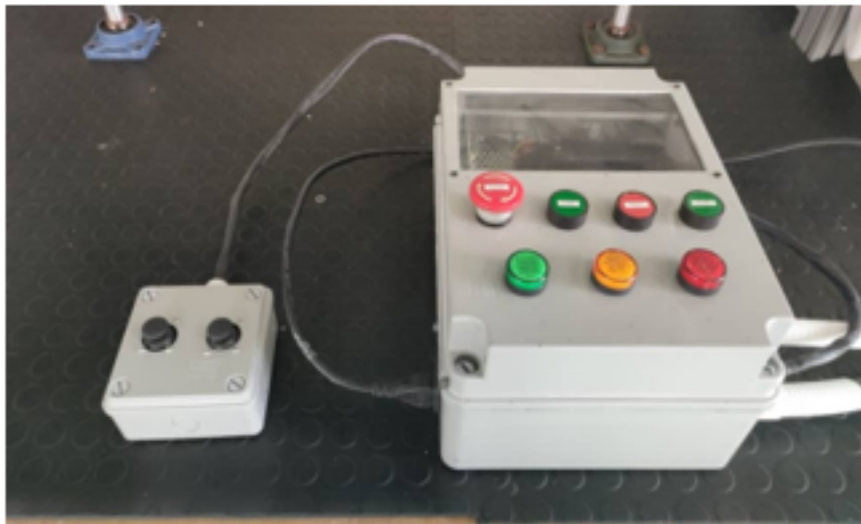
Figure 6: Joystick and PLC control box
