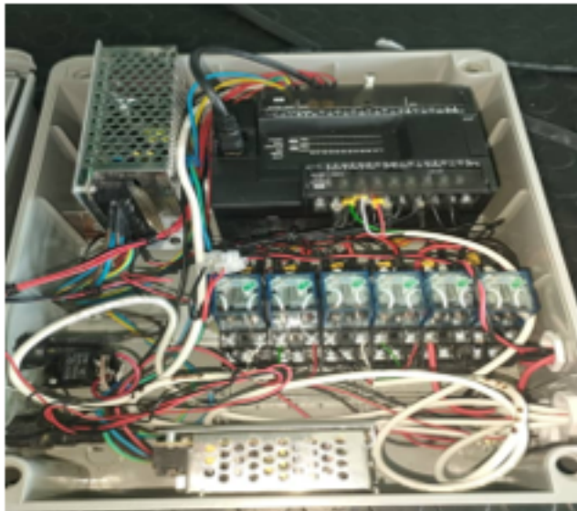
Figure 5: PLC and electronic components
